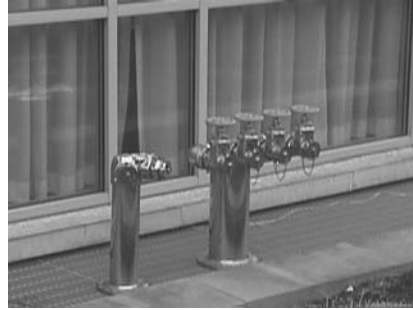
Figure 4.7. Siamese and Fire Pump Connection
