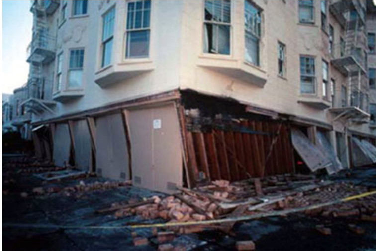
■ FIGURE 9.12 The first story of an apartment building in San Francisco, California, leaning to one side after the 1989 Loma Prieta earthquake. Courtesy of the U.S. Geological Survey.
