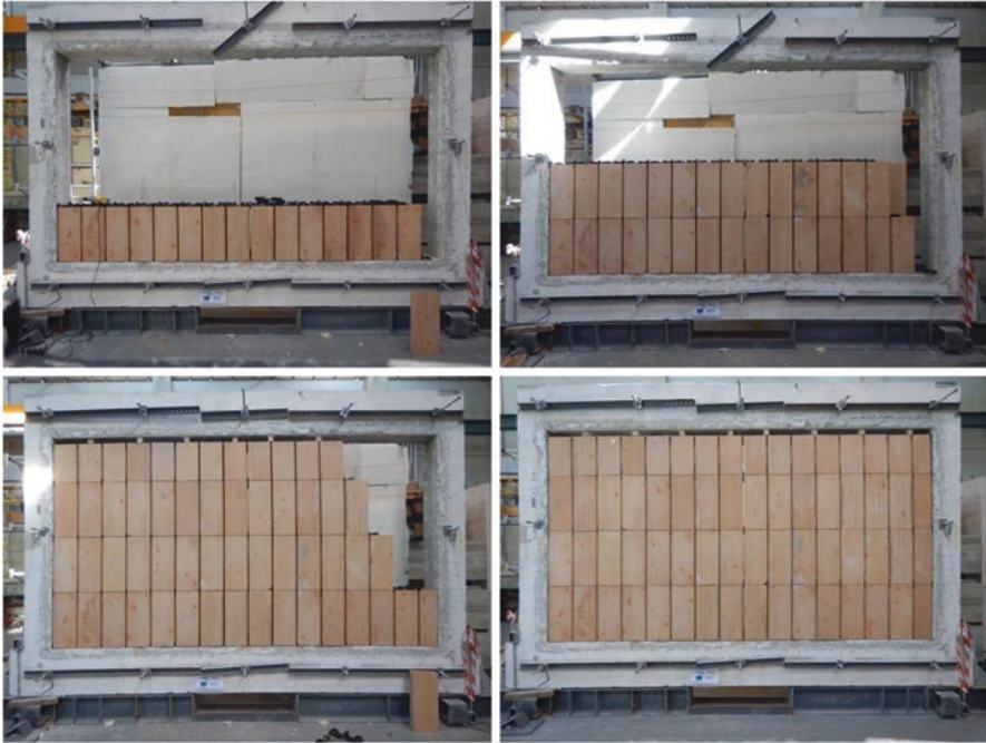
Fig. 12.3 Phases of assembly of first dry infill panel (from top-left to bottom-right picture)
