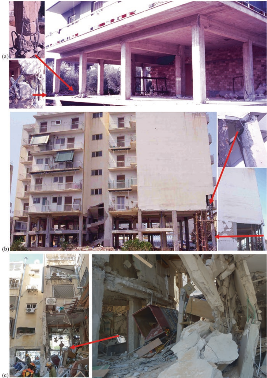
Fig. 2.17 Examples of upper floors working as cantilevering deep-beams with the infills in the role of the web, after loss of support due to (a), (b) the Kalamata, GR, 1986 earthquake; (c) gas explosion (Netanya, IL)
