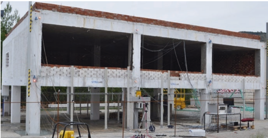
Fig. 2.20 Building without infills above the intermediate perimeter column removed in the final test phase
